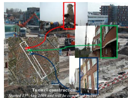
Figure 8. The locations for three PS points. The white rectangle is the area of ongoing tunnel construction. This tunnel construction started on 15 th August 2009 and will be completed in 2017
