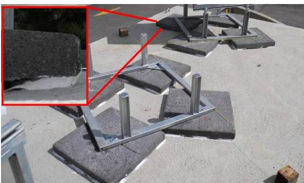
Figure 16. An example of the CR anchorage on the concrete surface. A particular of resin adhesive used to stick the weight on the roof, on the top right.
